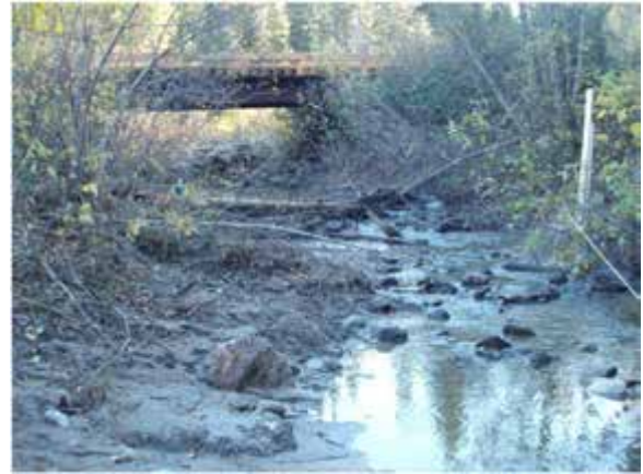
Upstream limit of affected area on Edney Creek (October 9, 2014).
