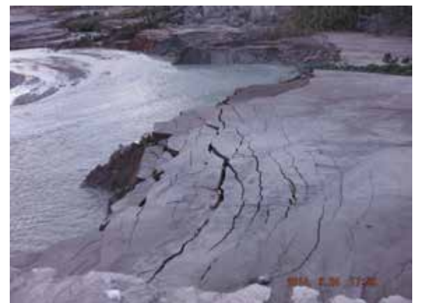
Downstream view of tension cracks in a sandy tailings deposit (September 24, 2014).
