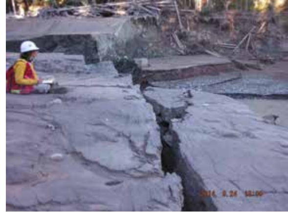
Tension cracks indicate a high potential for failure at the downstream extent of the entrenched section.
