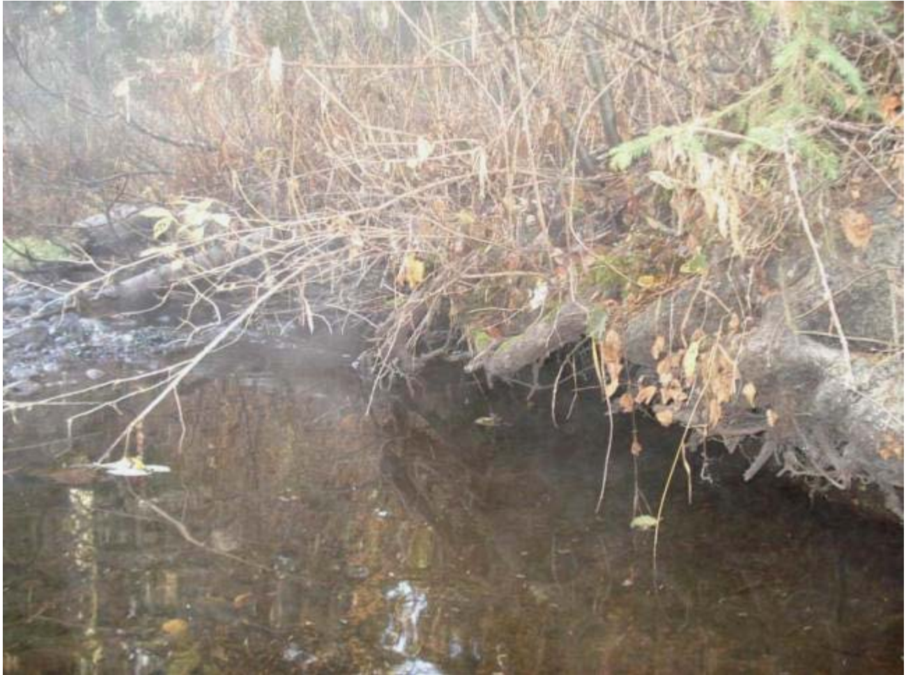
Figure 4-2: Undercut banks in reach four of Hazeltine Creek. Photo from Minnow (January 20, 2007)
