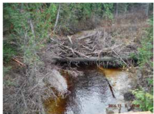
Upstream limit of affected area on Edney Creek. Photo taken upstream of the ditch road bridge (November 3, 2014).
