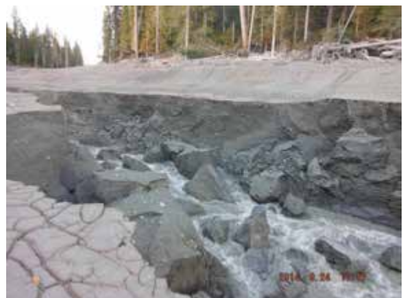
Channel incision into the thick lacustrine/glaciolacustrine deposit has led to rapid lateral erosion with calving blocks.
