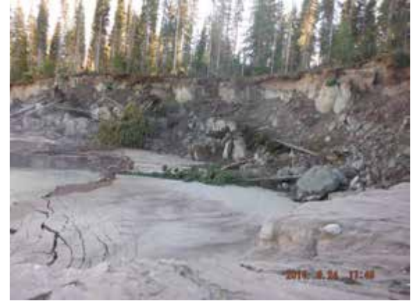
Failed sediment and vegetation along the right bank due to lateral bank erosion (September 24, 2014).
