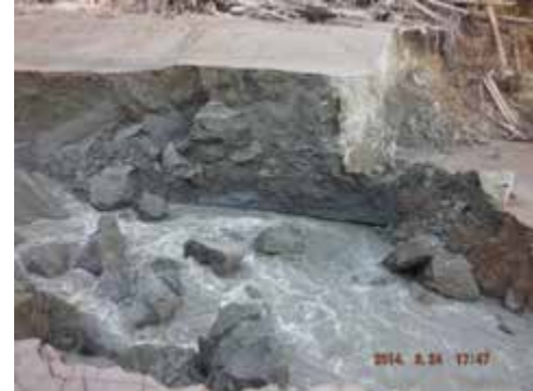
View of the left bank of Hazeltnine Creek. Large blocks of fine-grained native bank material have calved into the channel.
