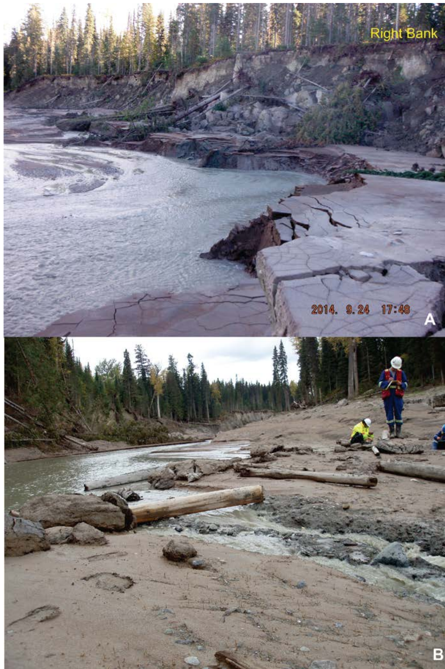
Figure 5-14: Slope failures at reach HC-R4a and HC-R4b. A- Figure shows extension of bank failures on right bank and location of sandy tailings. B – Figure shows extension of bank failures on left bank.
