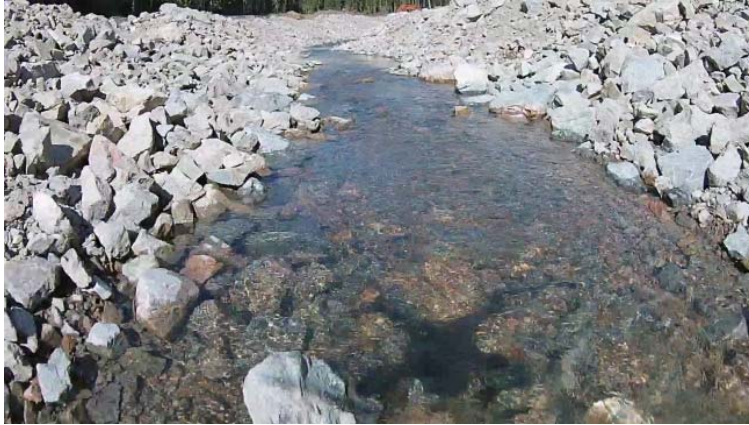
Figure 8. Hazeltine Creek turbidity has decreased since erosion control works, part of Hazeltine Creek channel rehabilitation, was completed on May 11, 2015.
