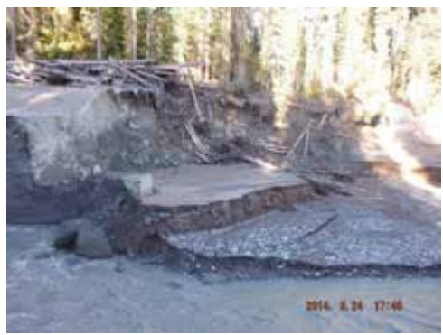
View of the downstream extent of a deeply entrenched section. Deposition has occurred where the channel widens.
