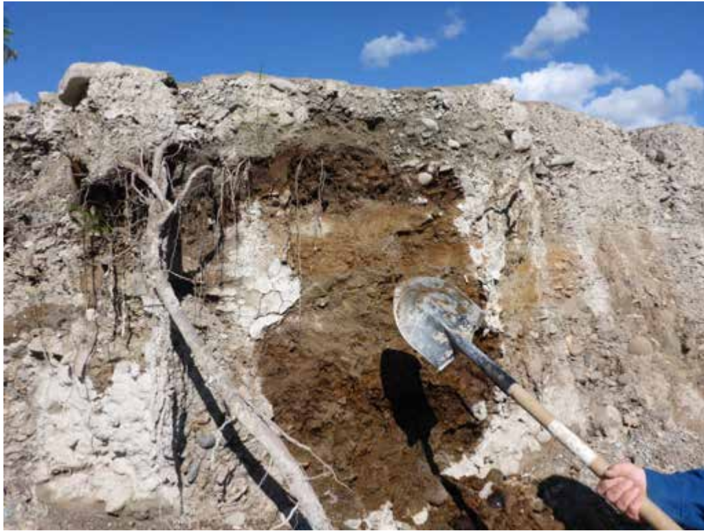
Photograph 13: View of ST02-07, showing a scoured sidewall soil profile in Lower Hazeltine Creek (September 3, 2014).
