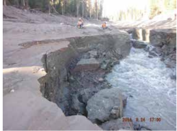
Large tension cracks form at the downstream extent of the lacustrine deposit.
