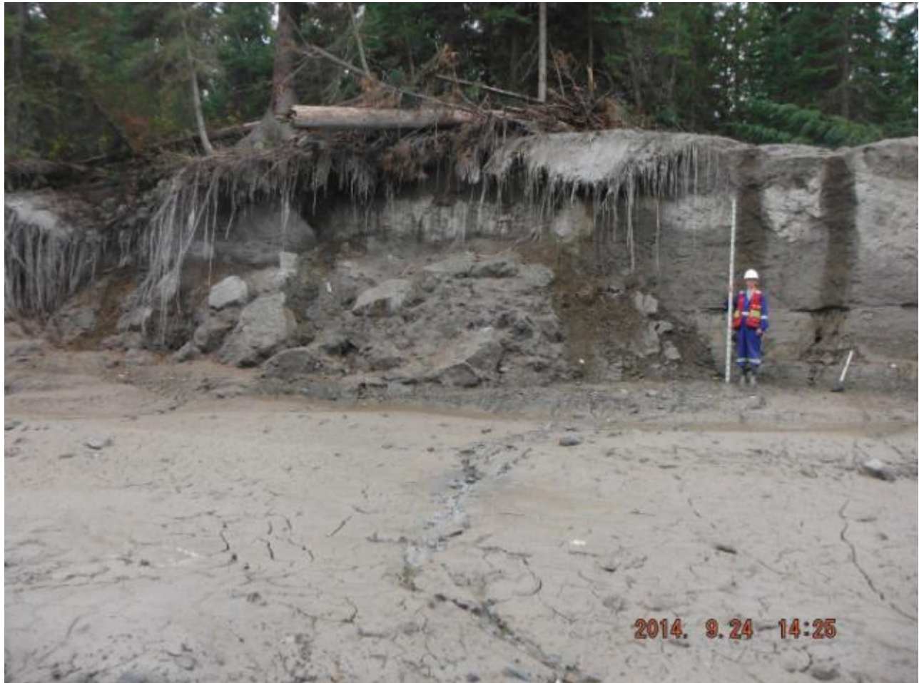
Figure 5-11: Eroded till zones within reach HC-R4a. Figure shows depth of scour and unstable slopes following the debris flow (September 24, 2014)
