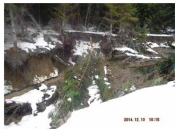
Channel incision and erosion of Edney Creek between the confluence with Hazeltine Creek and the ditch road bridge.
