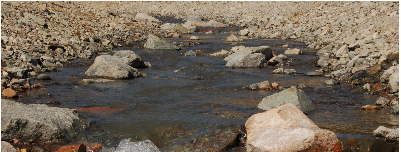
Lower Hazeltine Creek right after erosion control works in the channel had been completed. The water began to clear up quickly
