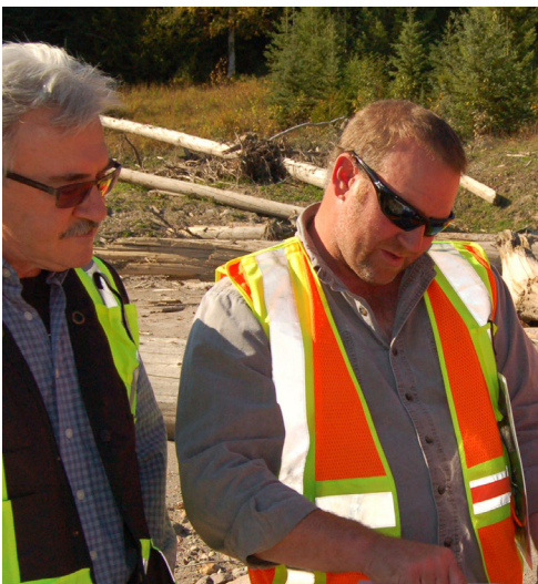
As soon as Hazeltine Creek could be safely accessed, construction works to control erosion were initiated
