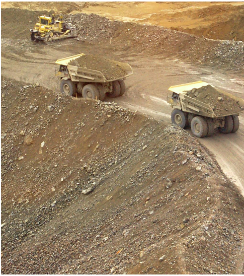
Haul trucks lined up to build a rock berm to hold back tailings in the TSF so that the breach could be repaired safely
